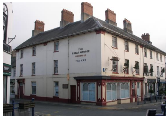
Fig.42 The Great George Hotel (corner Cross St & Monk St) an important high quality historic building in the townscape but much in need of repair and reuse.
