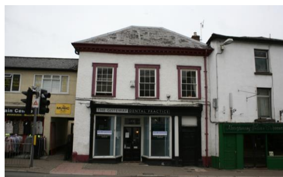
Fig.60 The vertical timber framed sliding sash, seen throughout the conservation area with various configurations of glazing bars – the example shown is a multi-paned sash window most commonly found in the historic core
